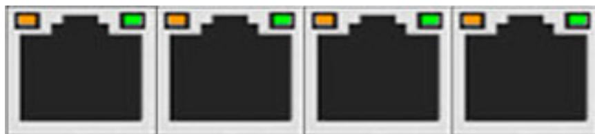
Fig. 4: Switch LEDs Switch LED indicators
